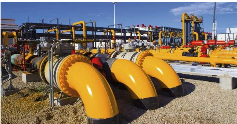
Fig. 96: Typical application field: gas compression station
